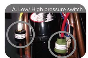
Low pressure switch High pressure switch
